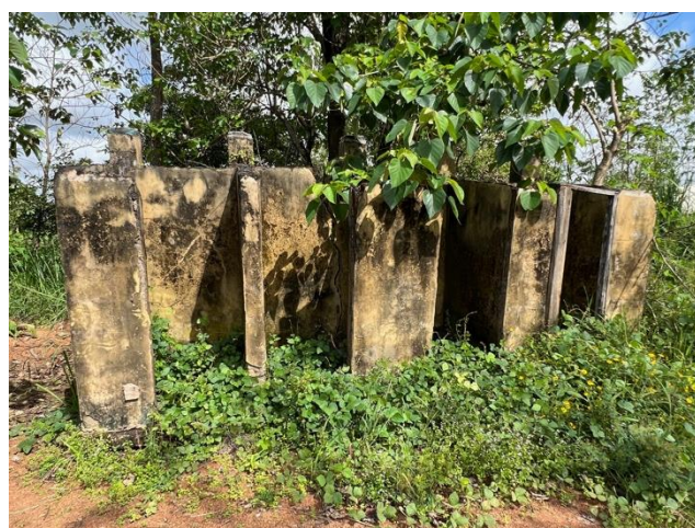
Prior to the Enviro Loo, these crumbling latrines were the only infrastructure available. Most students and staff avoided using them due to fear of snakes.
